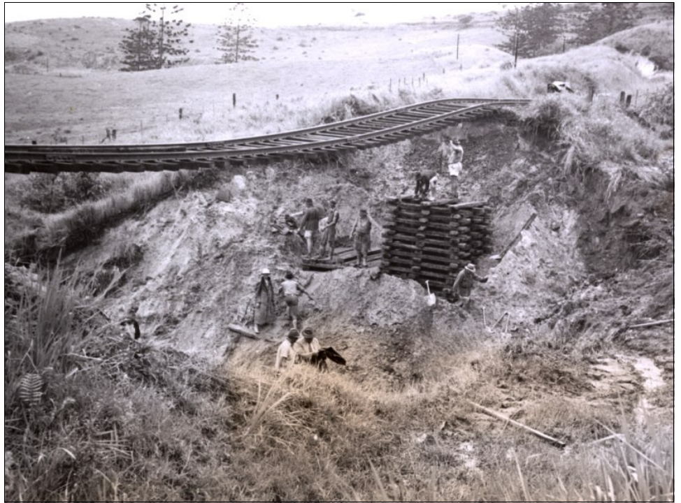
The tower of sleepers at the Casino end under construction. A considerable amount of earth had to be moved by men with shovels to form a flat base. SARA NRS 17420_2_1684_140G
