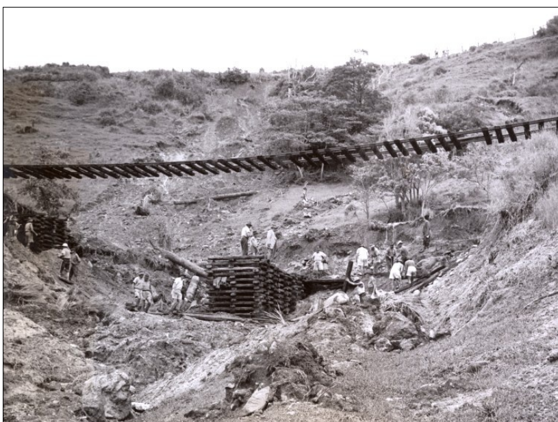
An early stage in the repair with the track still suspended over the missing embankment. Despite the previous wet spell the weather seems to have cleared to allow work to proceed in bright and dry conditions. SARA NRS 17420_2_1684_140H
