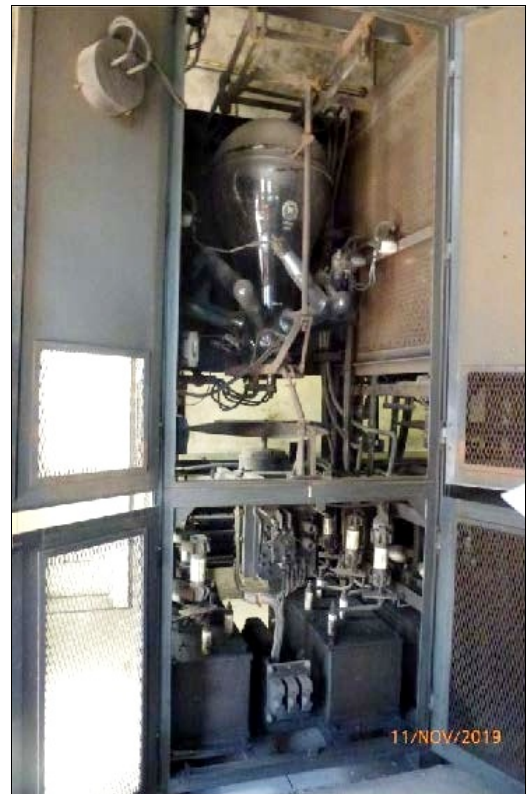
The 600 kW rated, Hewittic brand, mercury-arc rectifier bank has four, six-pole glass-bulbs each rated at 150 kW. Each bulb is housed in a dark grey painted, perforated sheet-steel cubicle, each with a propeller type metal cooling fan whose operating speed varies with the rectifier load current. This image (and caption), from Heritage Victoria, is of one of the cubicles with open doors, to show the rectifier and the fan.
