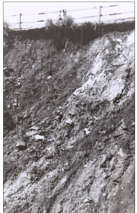
The original source of the landslide. The road may have avoided damage, but its future stability is precarious. SARA NRS 17420_2_1684_140B
