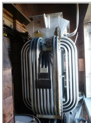
Side view of the Brunswick West rectifier transformer at the front door of the substation. Photo: Miles Pierce
