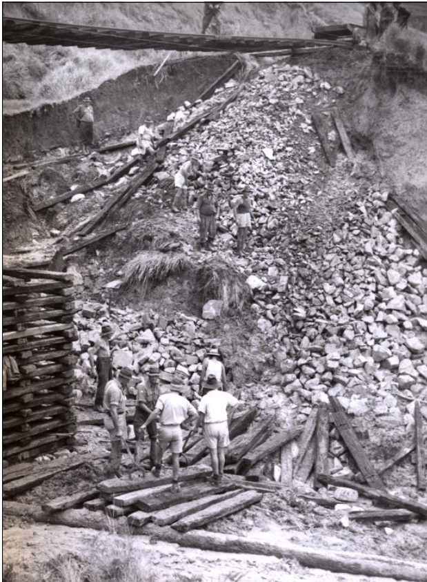
At the Casino end of the work the soil was seen as too soft, so spalls were dumped as a base for the tower. In the foreground the workers hold sleeper tongs, demonstrating the method by which the many heavy sleepers were manhandled into position. SARA NRS 17420_2_1684_140I
