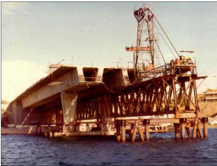
The Stirling Bridge – the Stage 1 upstream row (left) is completed, and the downstream row units are placed, but not stressed. Source: Don Young.
