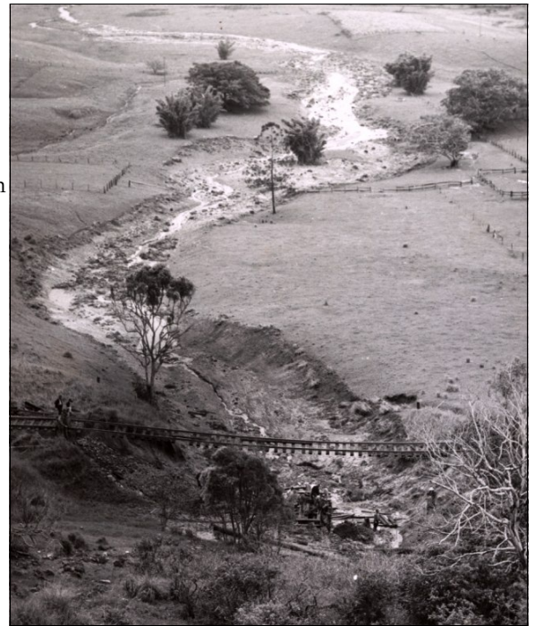
Viewed from the road above, the obliterated railway embankment and the extent of the mud flow beyond are clear. By this time, later on the day of the event, or the next day, workmen are already on-site starting repairs. The view here is from the west, looking toward the sea. - Murwillumbah to the left, Casino to the right. SARA NRS 17420_2_1684_140A
