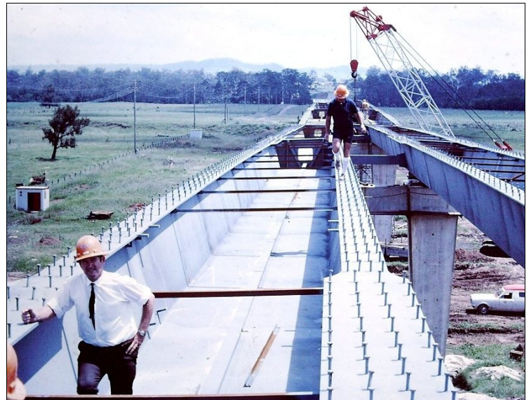
The Macarthur Bridge at Camden under construction circa 1972. Ray Wedgwood, Designer and Resident Engineer in the foreground. Photo: from Rob Wheen.
