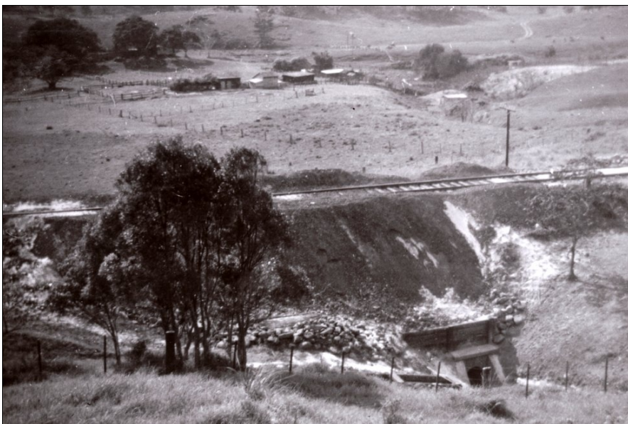
Deep in the gully, a substantial concrete culvert had been deeply buried by the landslide. The task of digging it out seems to have been left until the line was repaired and the embankment re-created. The re-exposed concrete culvert is seen at lower right in the photo. SARA NES17420_2_1684_140RB
