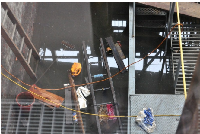
Flooding of the pump well nearly up to the operating floor in 2010, before work started on the pump house and before flooding was stopped. Image: Owen Peake.
