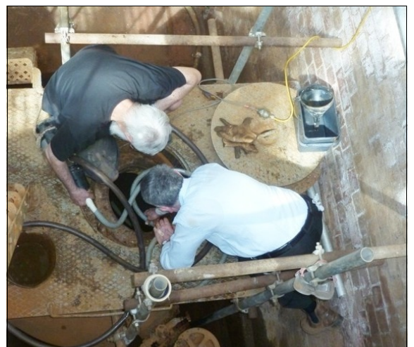
The author & Derek Moore pumping flood water from a pump casing. Image: Miles Pierce, Sept. 2013.
