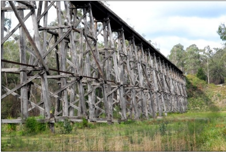
The Stony Creek railway viaduct near Nowa Nowa, Victoria. Image: Owen Peake
