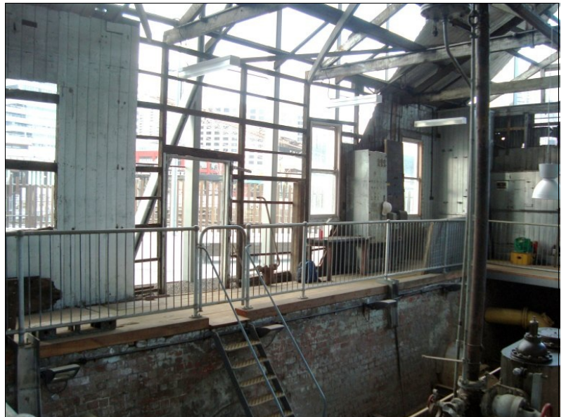
From the inside looking out. Shows the fence around the pump well with gate & ladder. The steam engine cylinder is at bottom right. Through the glass there are glimpses of the tall buildings on the other side of the Yarra. Image: Owen Peake 10 Sept 2013.
