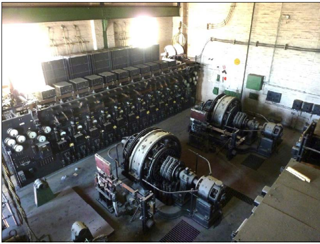
Rotary converters, installed in a Melbourne Tram Substation in c1929. Decommissioned in the 1990s, but still in situ. Photo: Miles Pierce.
