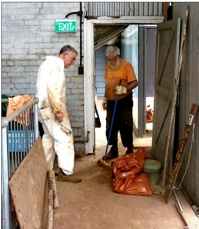
The author (right) and Derek Moore clean the concrete ground floor around the pump well prior to repainting it.
