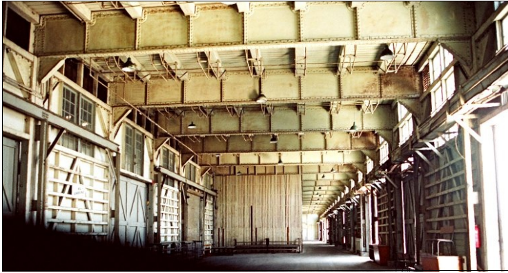
Typical wharf shed interior, possibly 9, looking south. Shows underside of the upper floor structure, described at right. Image: M.Doring, December 1987.
